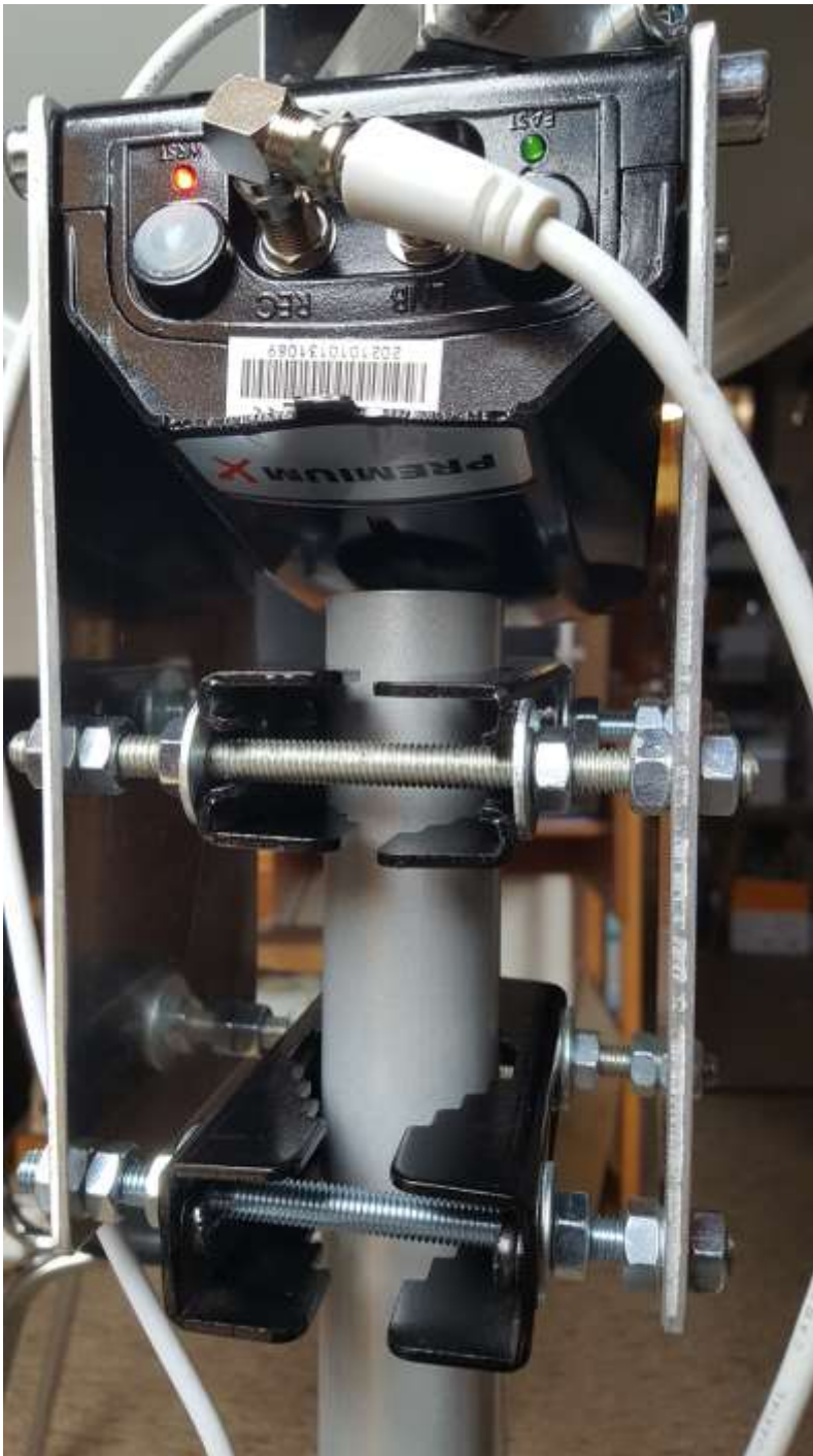
Figure 2 ~ Detail view of the azimuth rotor fixation on top of the tripod pole.
