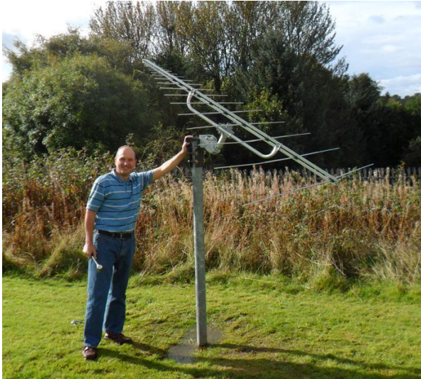
Figure 16 ~ Log periodic dipole array antenna (LPDA) mounted on a mast with a rotator and low noise amplifier. The 21-element Creative Design CLP5130-1N antenna frequency range is 50 to 1300 MHz and its free space gain is 6 to 8 dB. This antenna installation has a fixed elevation but can be turned to any hour angle with the rotator. The low noise amplifier has a noise figure of about 1.0 dB and a gain of about 20 dB. Setup at University of Glasgow, UK. Image ©2012 C. Monstein.
