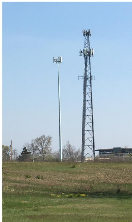
Figure 5: Cell Towers Producing LNA Overload
