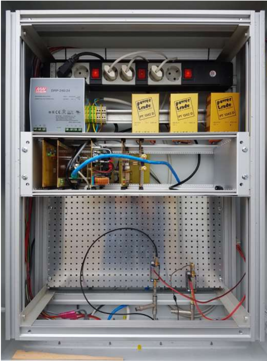
Fig 4: Setup of outdoor cabinet
