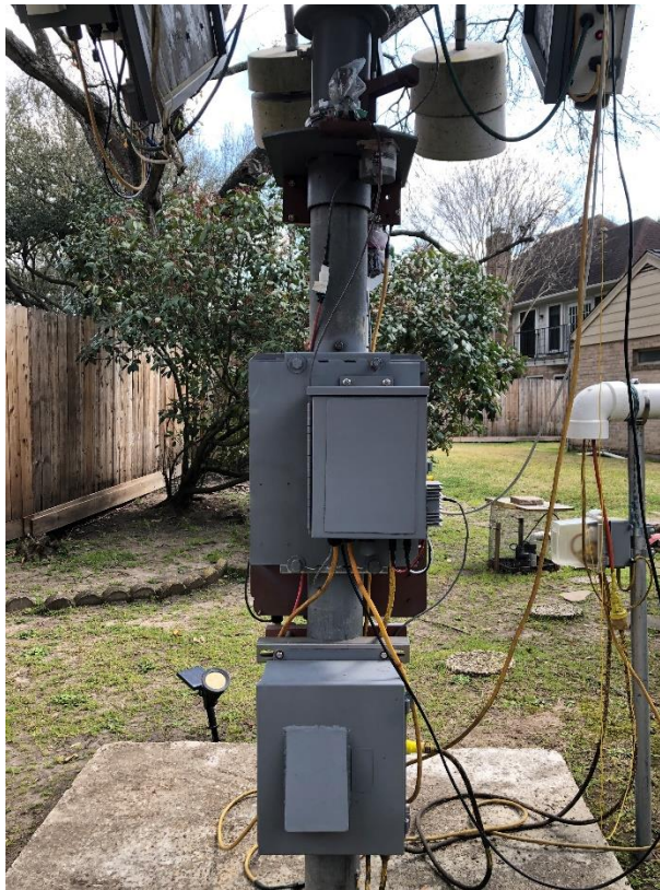
Figure 1: Motor and Speed Control Hardware Mounting
